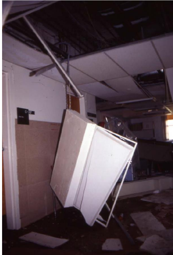
Photo: Light fixture dangling from conduit following the 1994 Northridge earthquake, U.S.A. Source: FEMA E-74, January 2011, Reducing the Risks of Non-structural Earthquake Damage – A Practical Guide.
