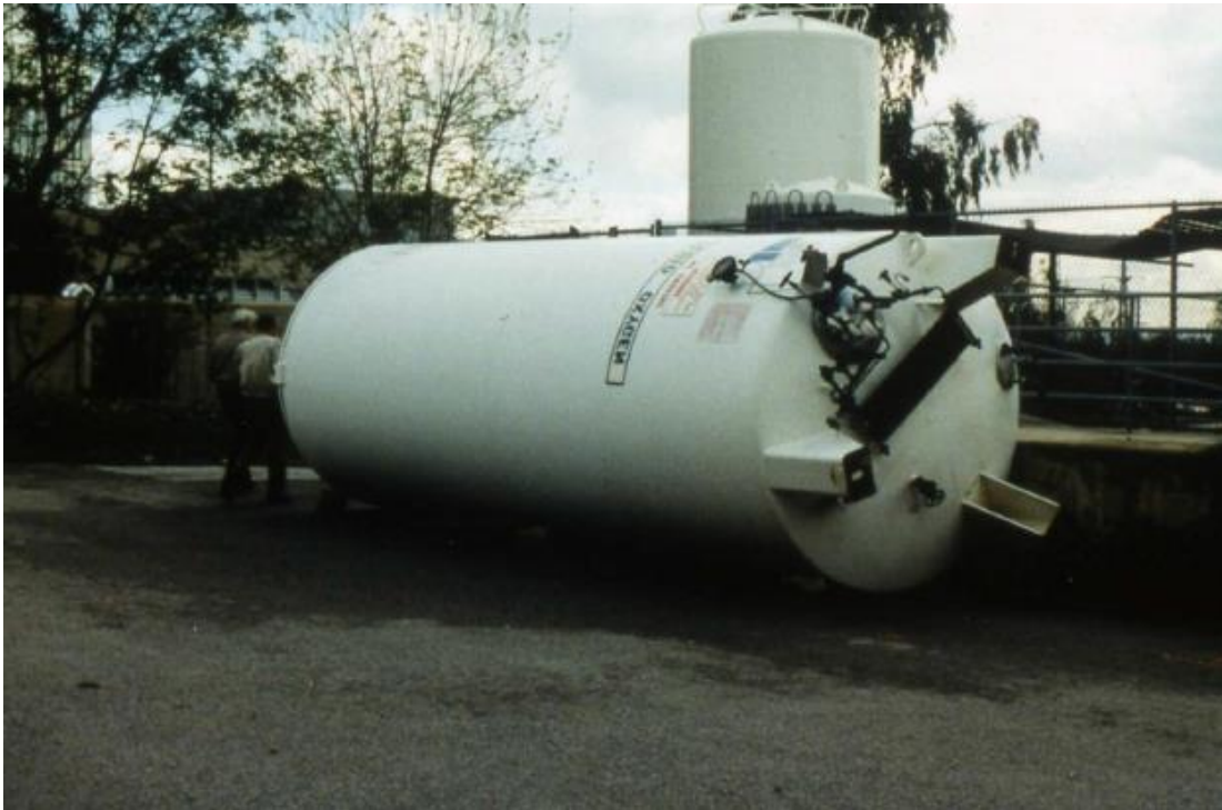
Photo: A vertical tank overturned in the 1994 Northridge earthquake, U.S.A. Source: FEMA E-74, January 2011, Reducing the Risks of Non-structural Earthquake Damage – A Practical Guide.
