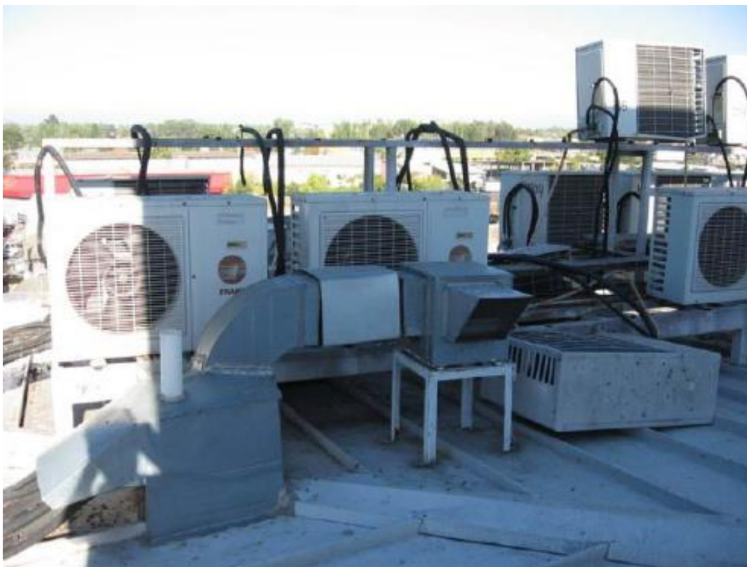
Photo: Topped air-conditioning units following the 2010 Chile earthquake. Source: FEMA E-74, January 2011, Reducing the Risks of Non-structural Earthquake Damage – A Practical Guide.
