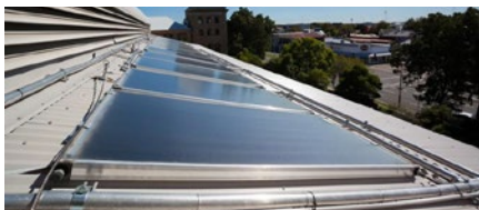
Flat plate solar panels installed on TAFE site roof
