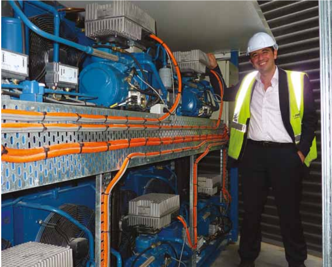
Inside the plant room.
