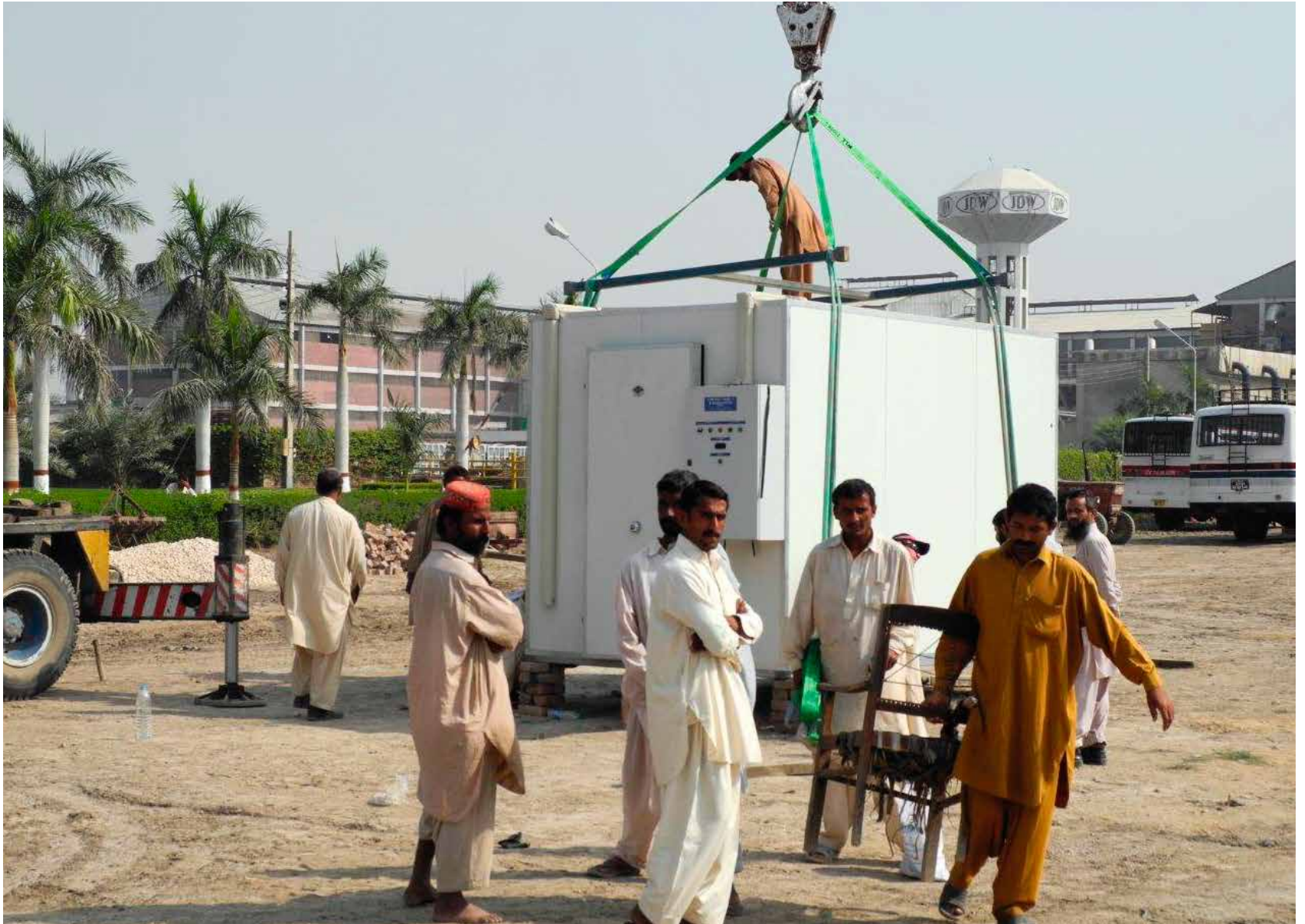
On-site at JDW Sugar Mills – one of Pakistan's largest sugar cane producers.
