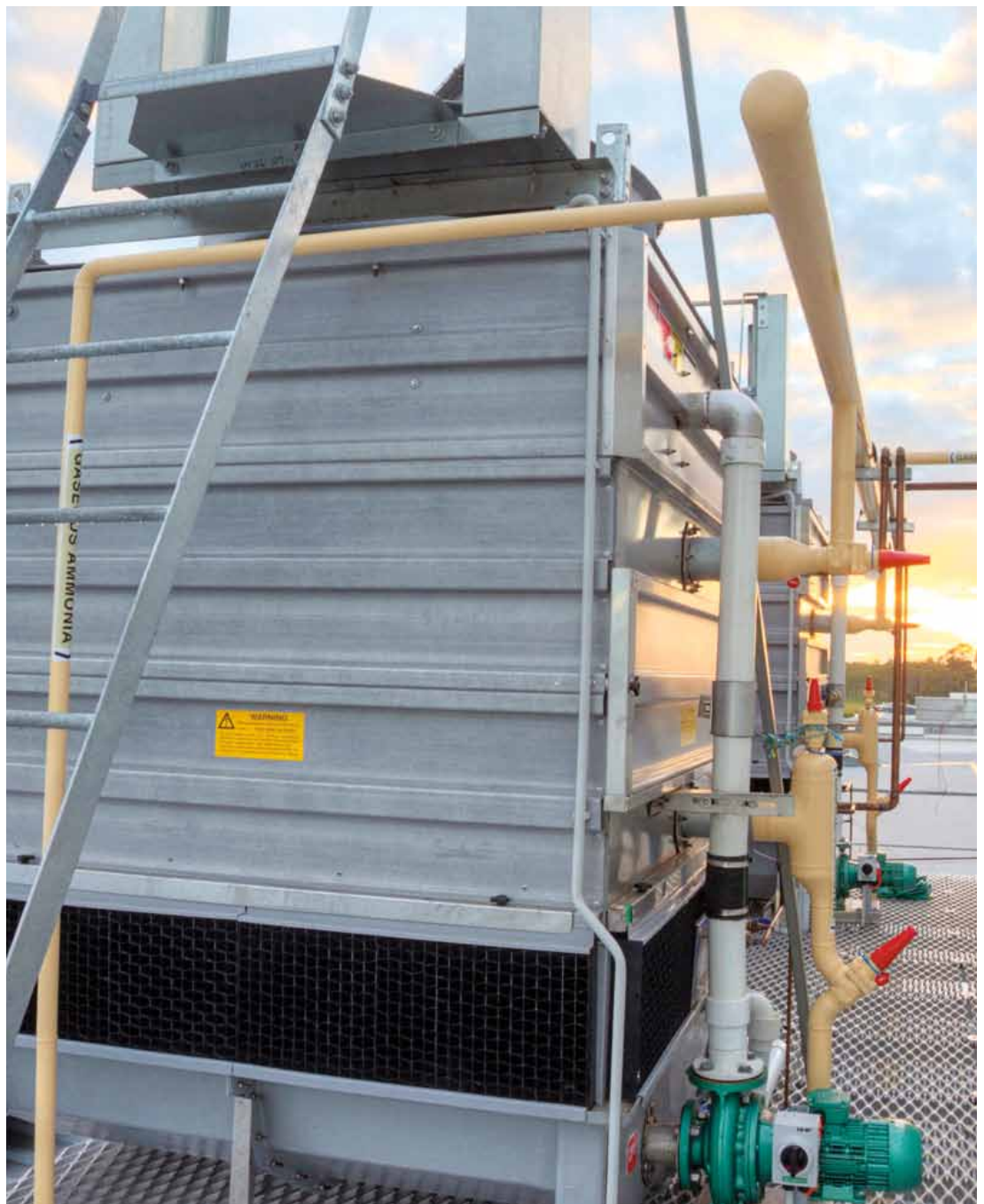
Condensors on the roof of the new fit-out.
