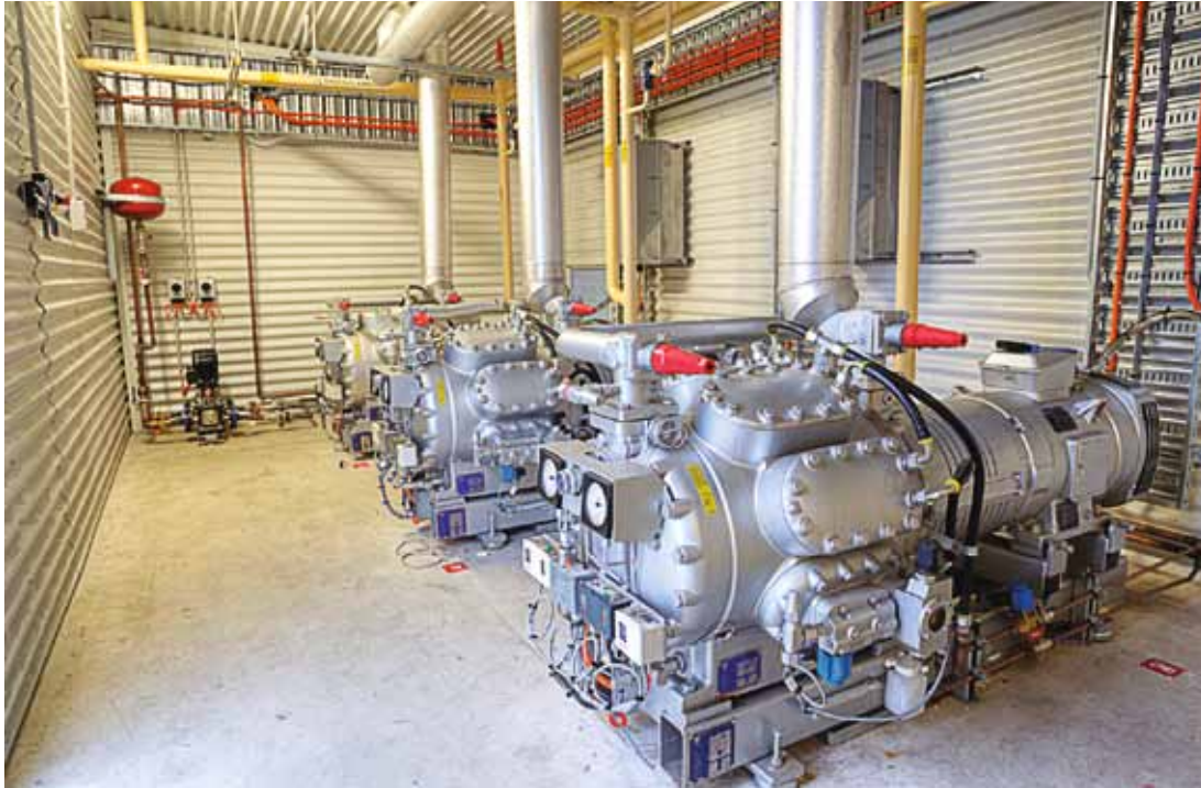
Compressors inside the plant room at Richmond Dairies, Casino.
