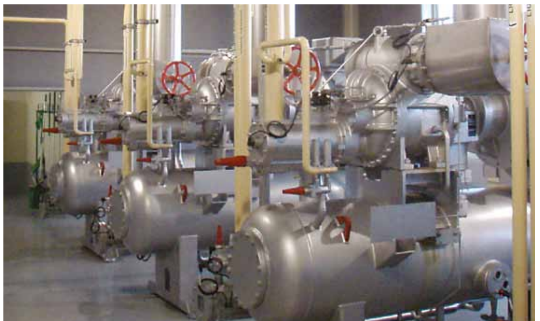
Inside the plant room.
