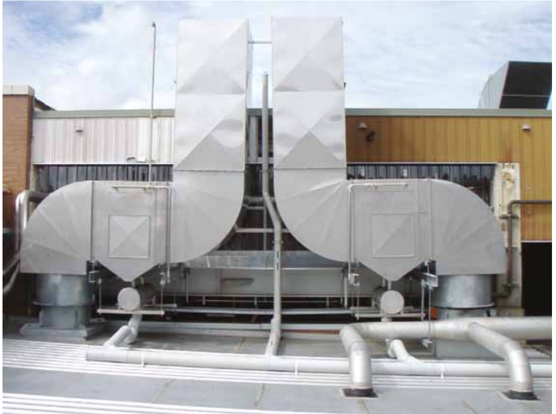
Scrubbers on the brewery's exterior.
