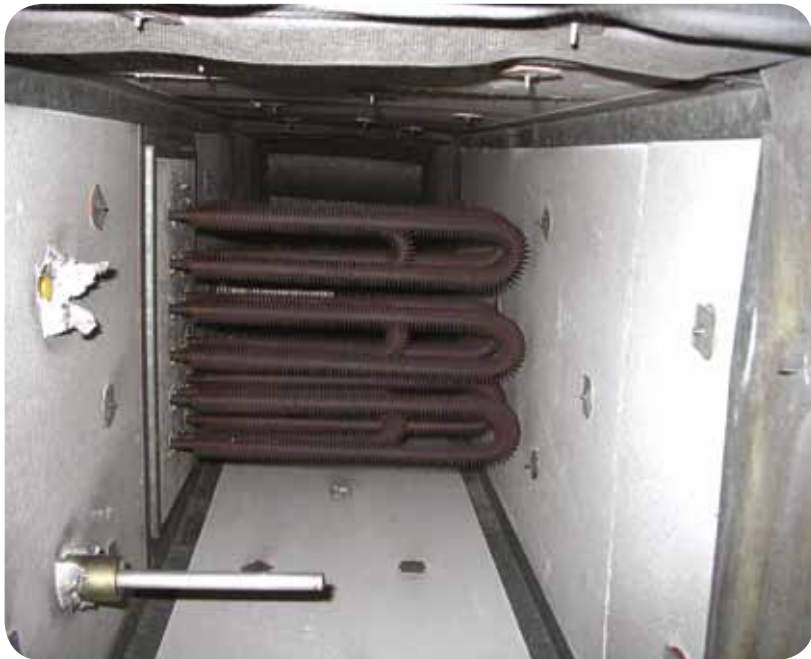
Asbestos lining within a heater bank.
