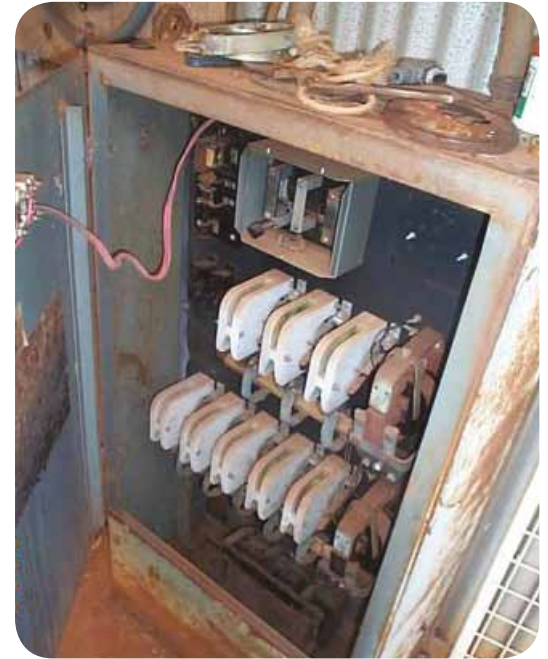
Mechanical switchboard with ceramic fuses.
