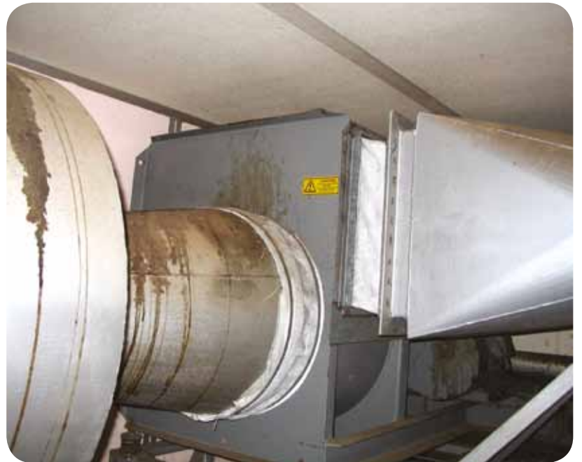
Textile flexible joint in the exhaust duct.
