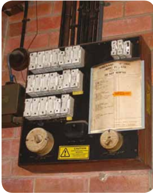
Typical old-style switchboard with ceramic fuses.
