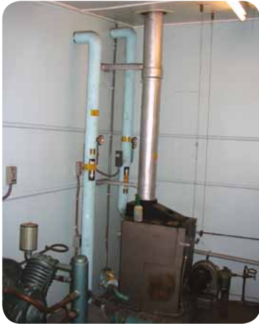
Oil burner heater.
