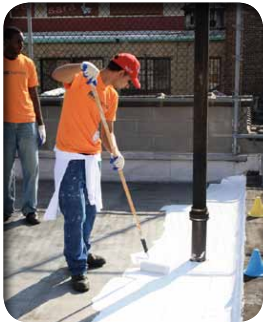
New York City's rooftops are being covered in a special cool roof coating.
