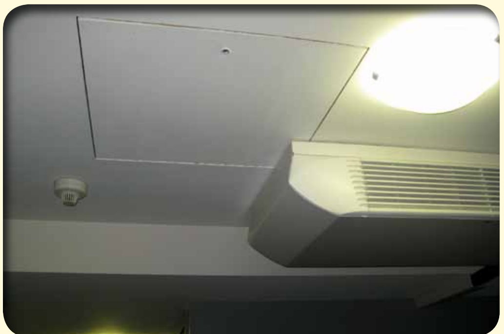
Another poor example of restricted access.
