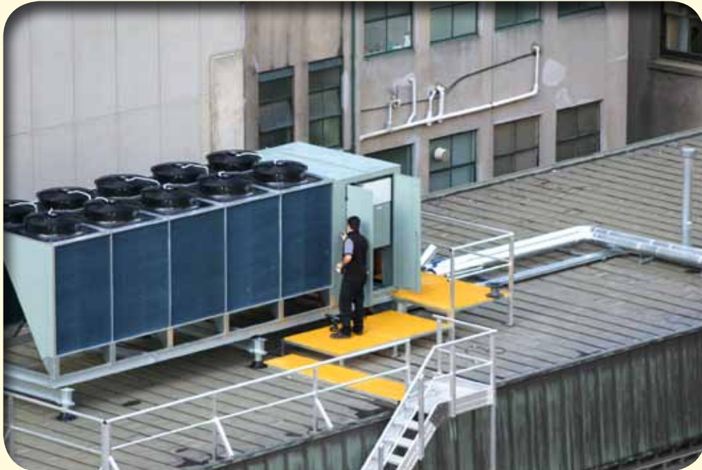
An example of the use of fixed platforms, walkways and stairways.
