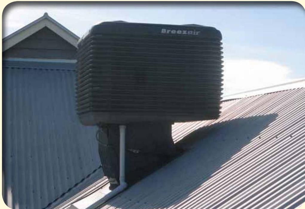
Evaporative cooler outdoor unit.
