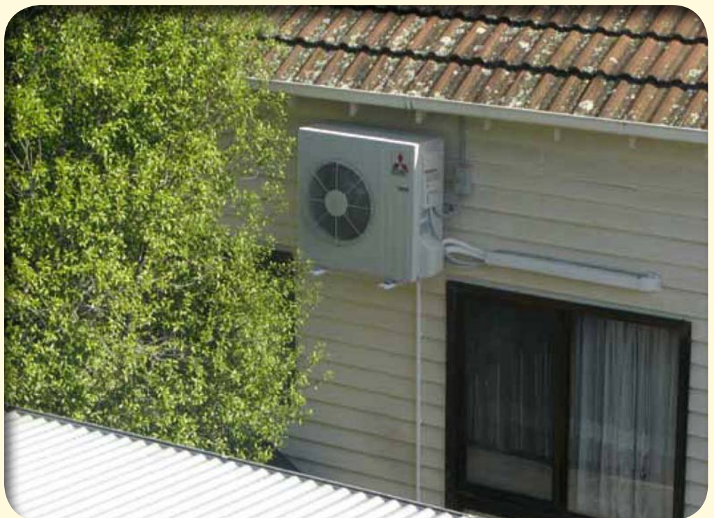
Split system outdoor unit.
