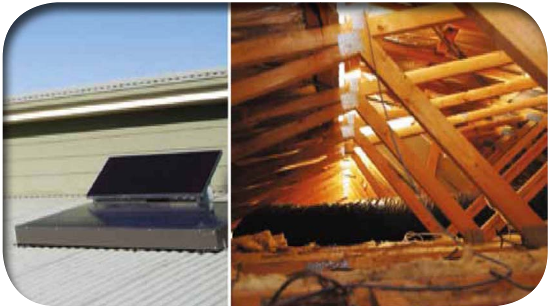
Solar air heater on the roof of the Selwyn Neighbourhood House, with the duct located in the roof space.
