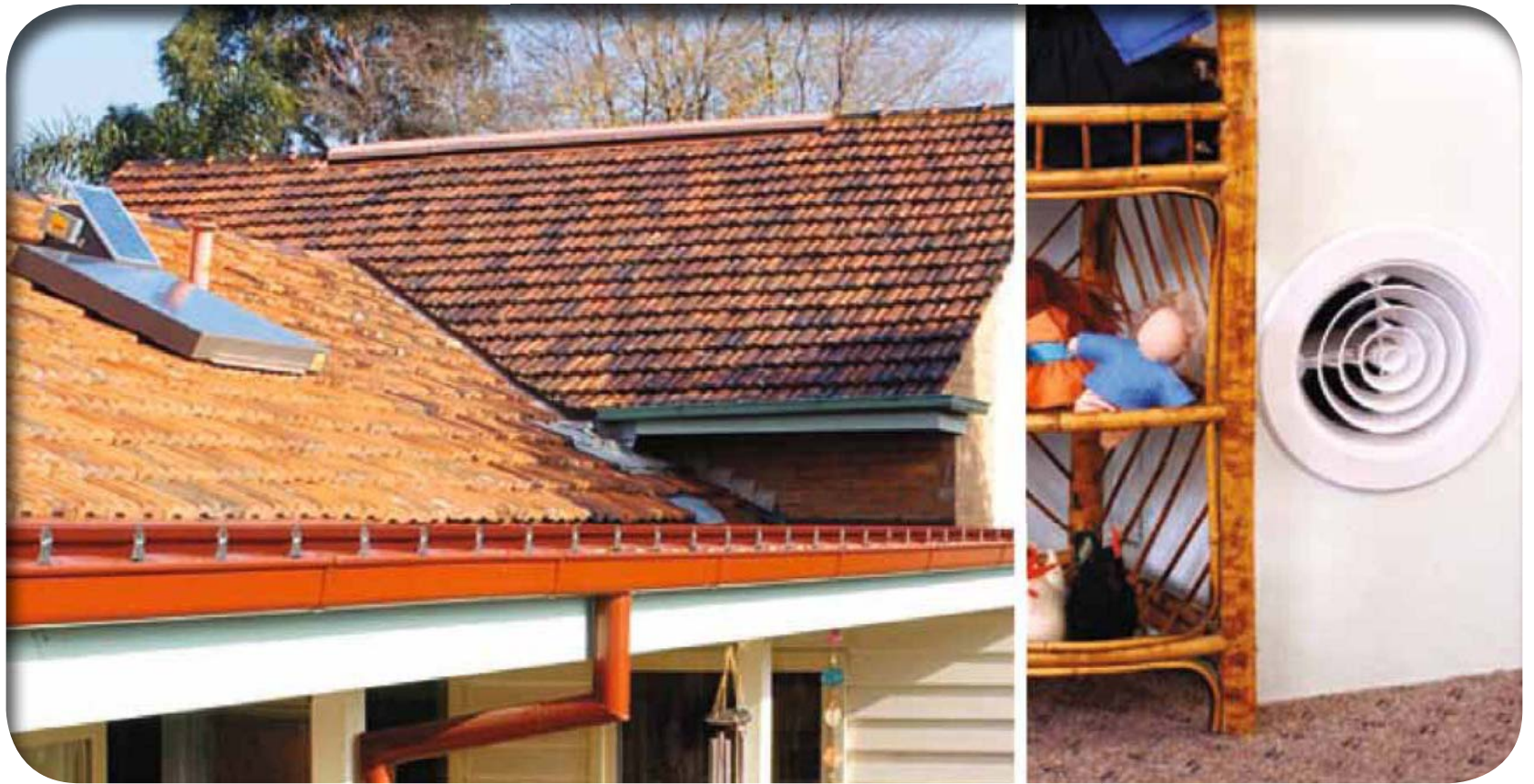
Solar air heater on the roof of the Audrey Brooks Memorial Pre-school, and internal outlet vent in the main classroom.
