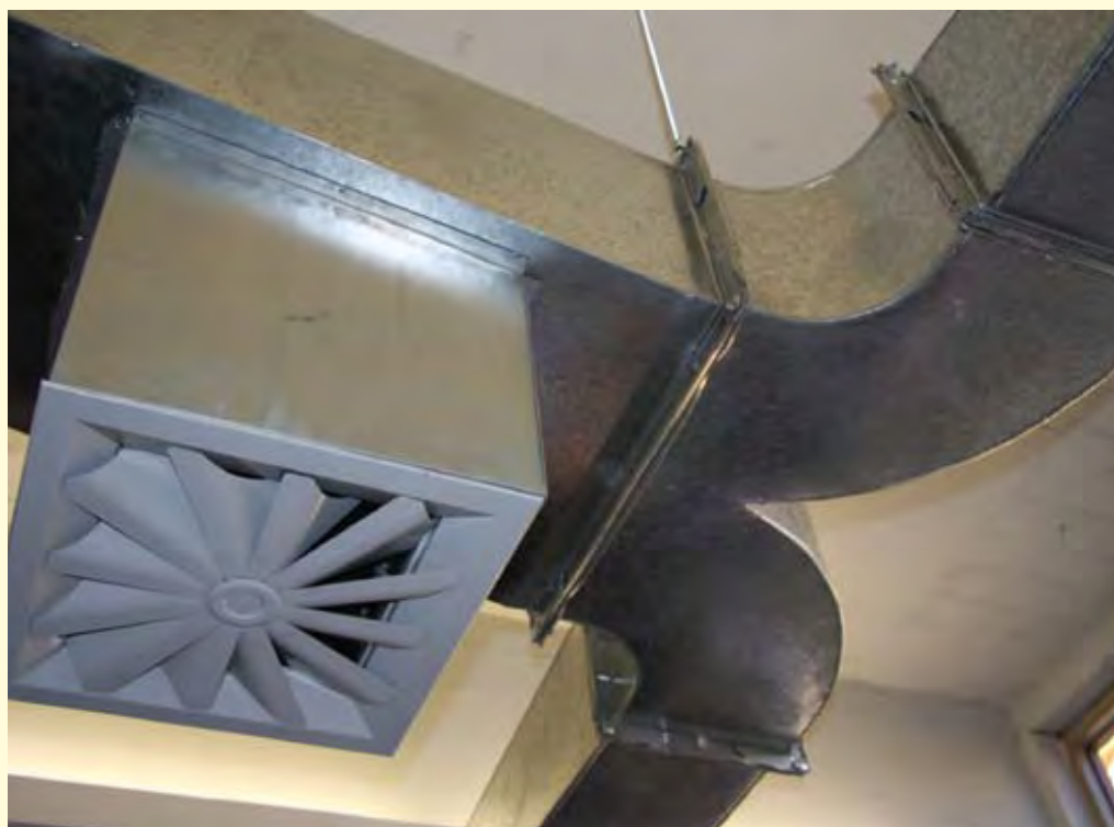
Exposed office ductwork
