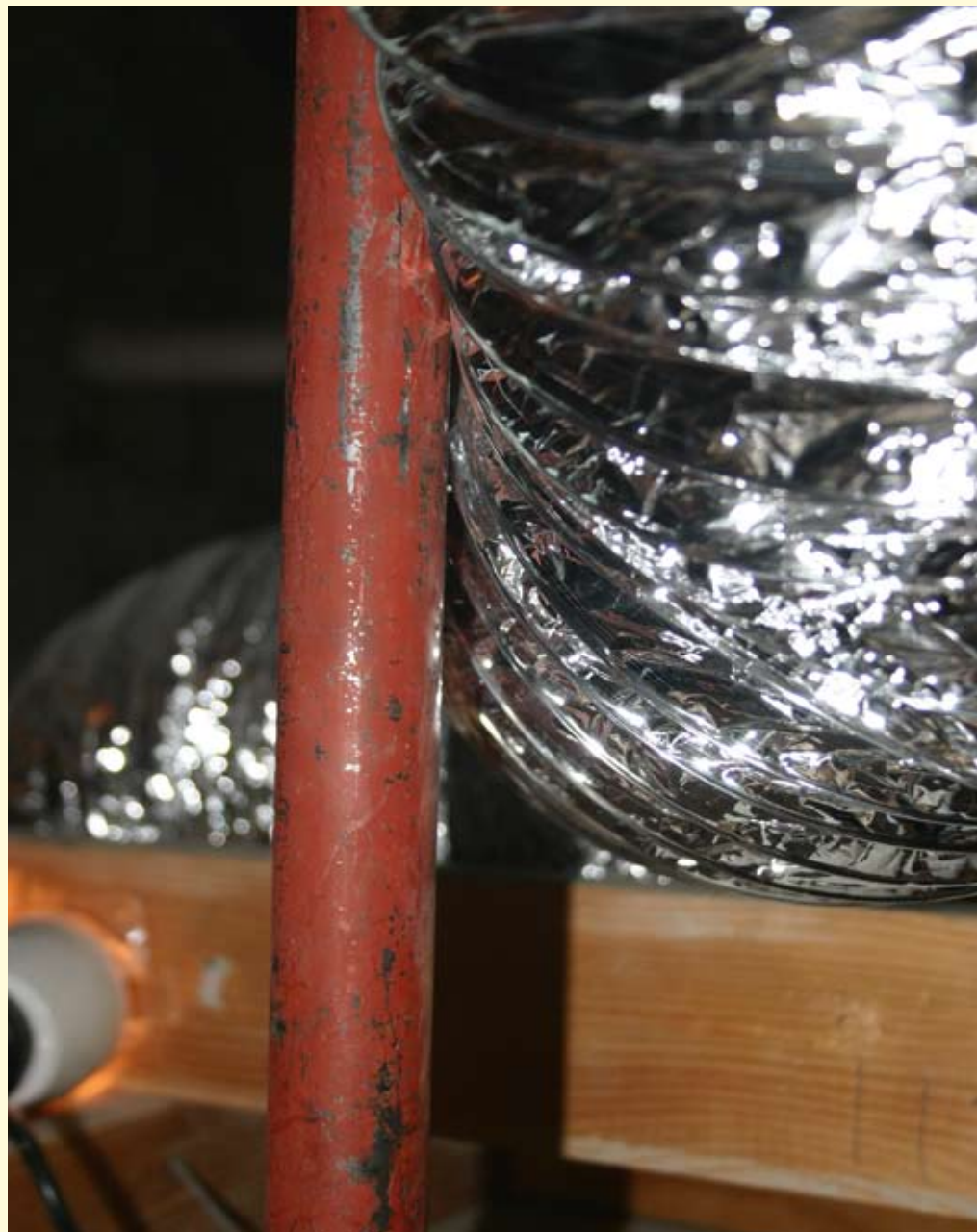
Duct clashing with other services.
