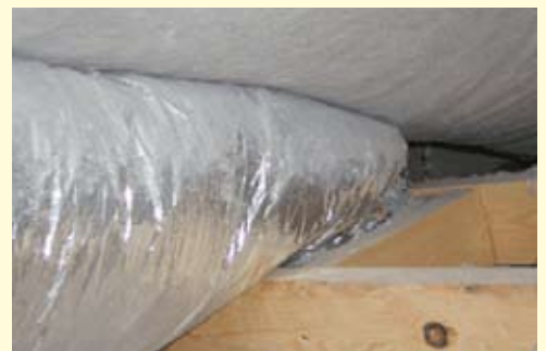
Duct constricted by bend into boot.
