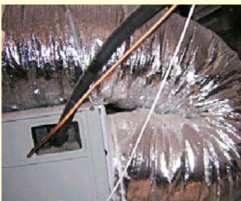
Radius of bend less than one-duct diameter.
