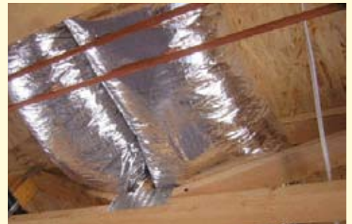
Ducts compressed into small space.
