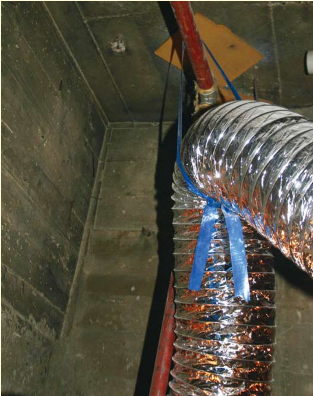
Inappropriate support and restricted bend.
