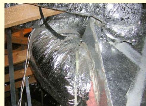
Duct constricted by bend leaving plenum.
