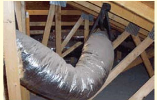
Improper duct support and excess duct sag.
