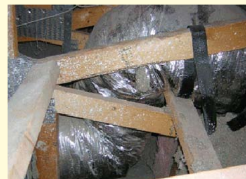
Duct constricted by two bends leaving plenum.
