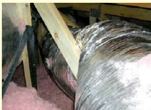
Duct constricted by bend over truss web.
