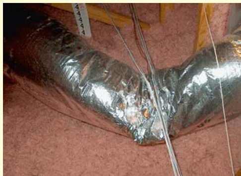
Duct compressed by wires.
