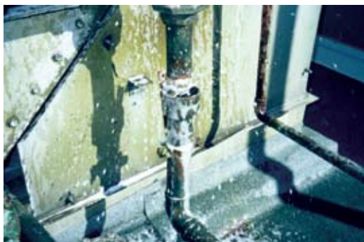
Figure 2. Tower overflowing with chemical loss
