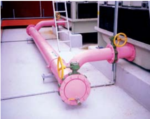
Fig 5. Balance line too low, should be located at basin sump height.
