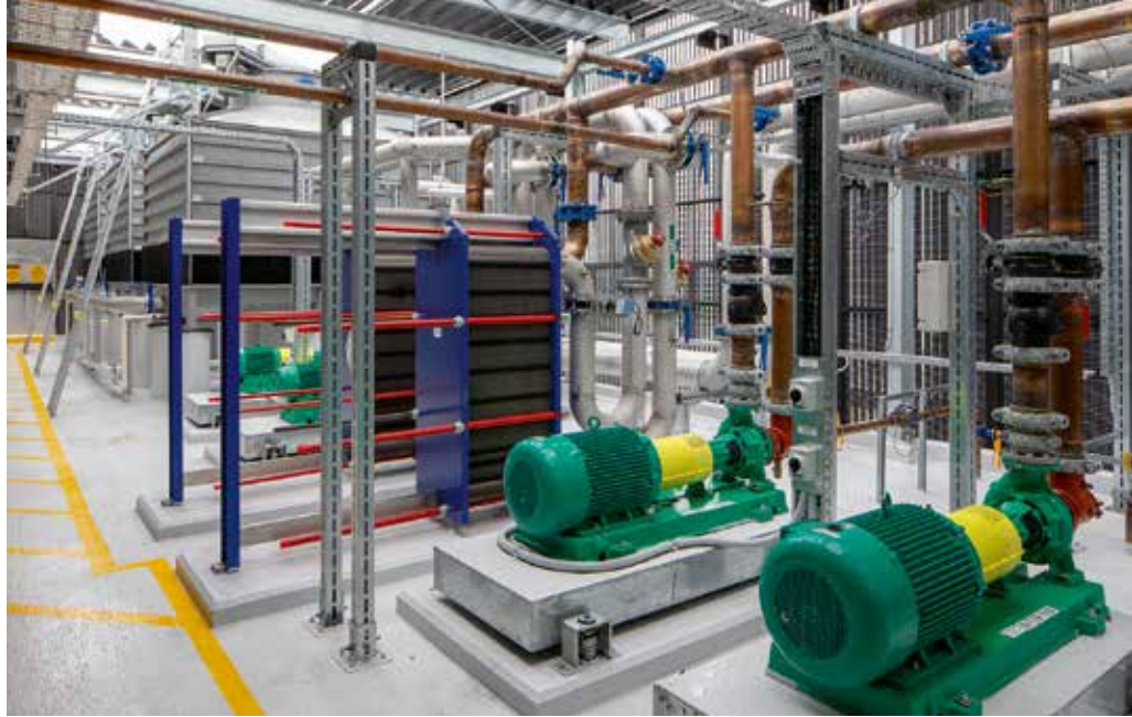
Cooling plant consists of two equal-sized chillers served by three equal-sized cooling towers. Image courtesy of A.G. Coombs.
