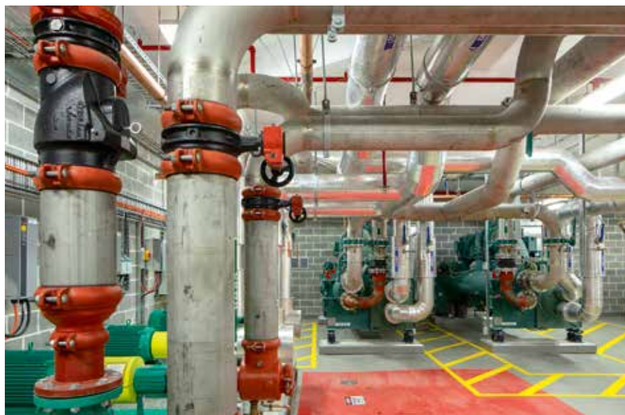
Very exacting levels of installation accuracy were required to closely match the detailed 3D model, these were delivered using BIM-to-laser set out methods. Image courtesy of A.G. Coombs.
