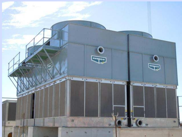
Counter flow induced draft cooling tower
