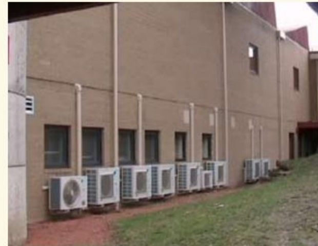
Air-conditioning systems located at ground level with good access.
