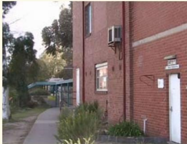
Air-conditioning system high on a wall in a commercial setting.
