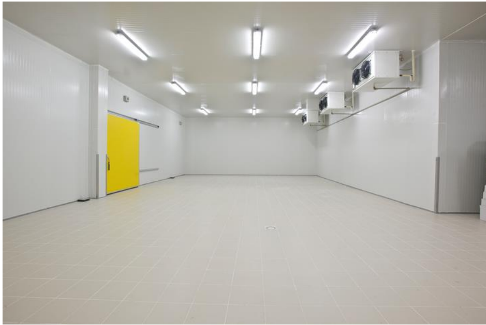
Figure 1: New walk in cool room with three evaporators.
