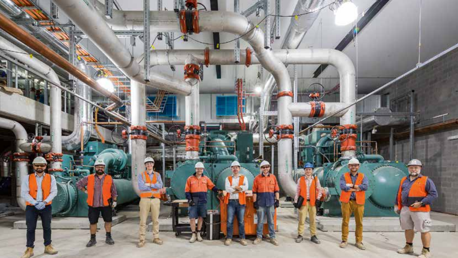
The chilled-water plant consists of six high-efficiency centrifugal water-cooled chillers.
