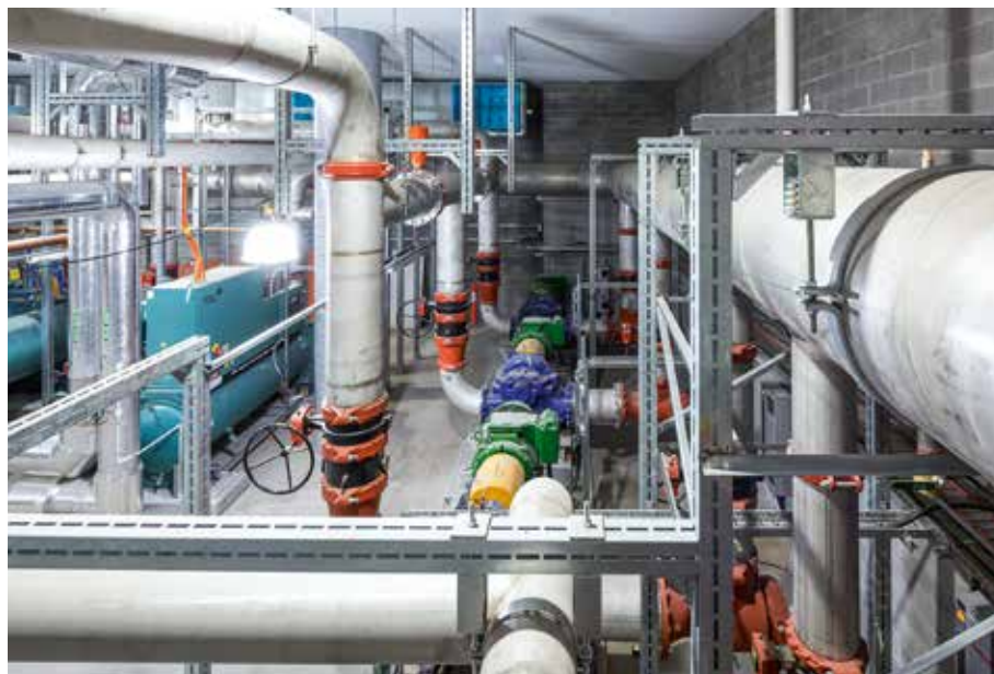
The central plant solution offered better piping efficiency, more flexibility for plant selection and optimisation, and better accessibility and maintainability.
