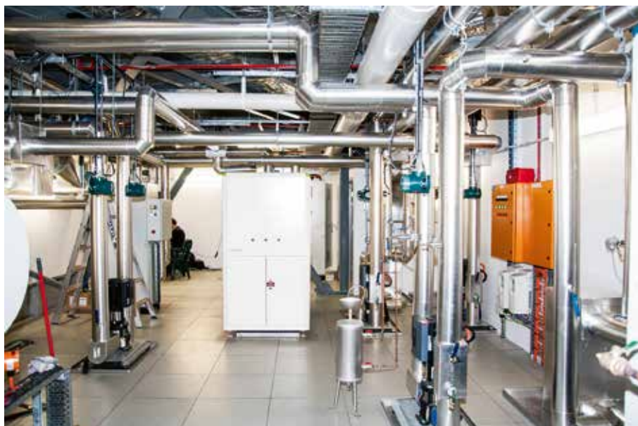
The plant room during commissioning. The ORC (Organic Rankin Cycle) is front and centre.
