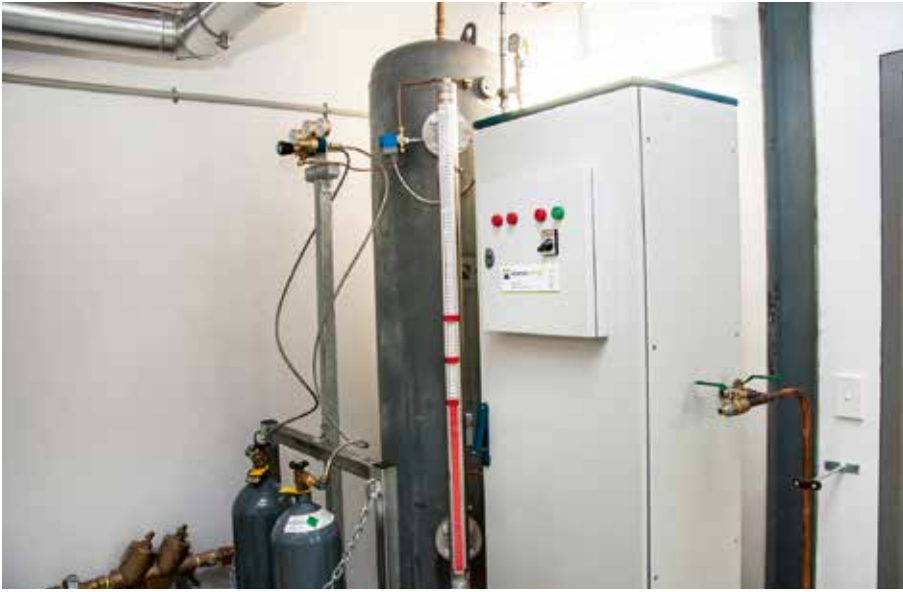
The fluid thermal expansion system is suitable for high temperatures. A nitrogen blanket is used.
