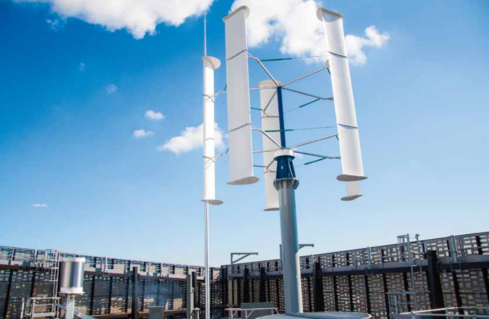
The vertical-axis wind turbine charging a flow battery.
