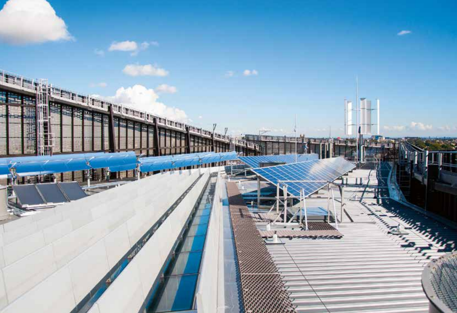
There are our new energy technologies on the roof: solar parabolic collectors, flat-plate collectors, PV, and wind turbines.
